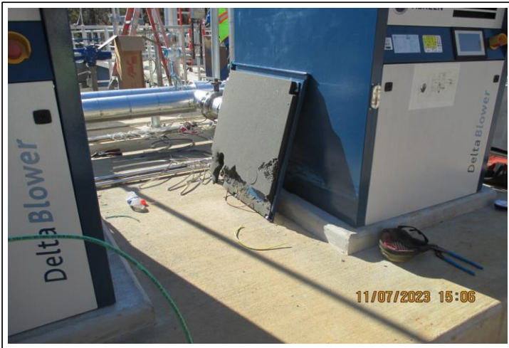
Rodent Damage to the UV Blower Insulation Panel
