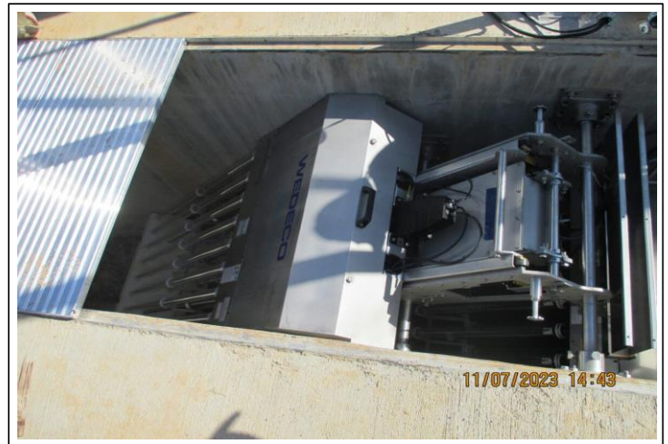
UV Disinfection Light Banks
